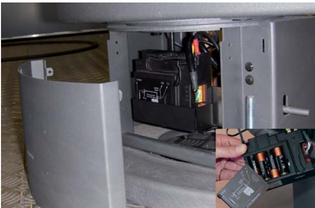
Replacing the batteries of the receiver.
