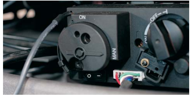
The gas control switch
